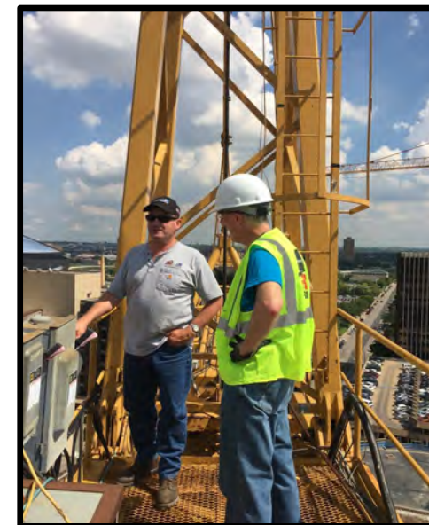
Tower Crane Operator, Tim Olson and Dr. Jon Pryor taking in the view from the deck of the tower crane.
