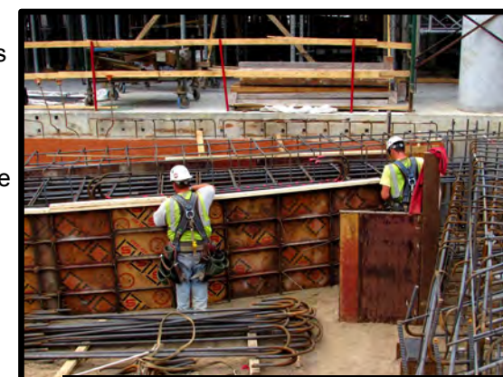
Various sizes and weights of rebar used to reinforce concrete structures throughout the building
